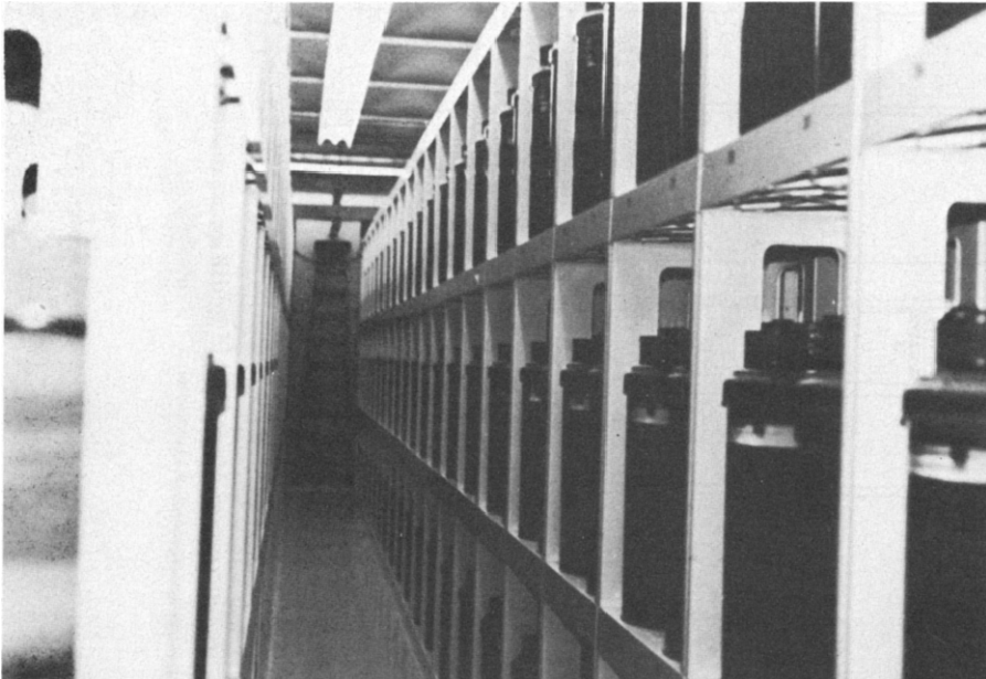
Fig. 9. Portion of a 2 000 kV A battery plant.
